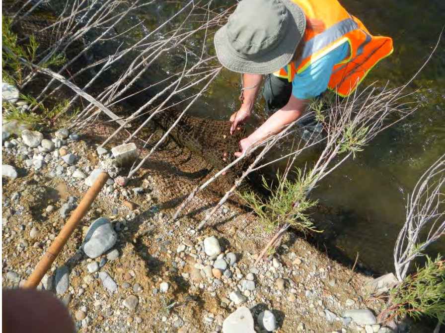
Photo 10. Torn fabric on slumping DVSL, Phase 1.
