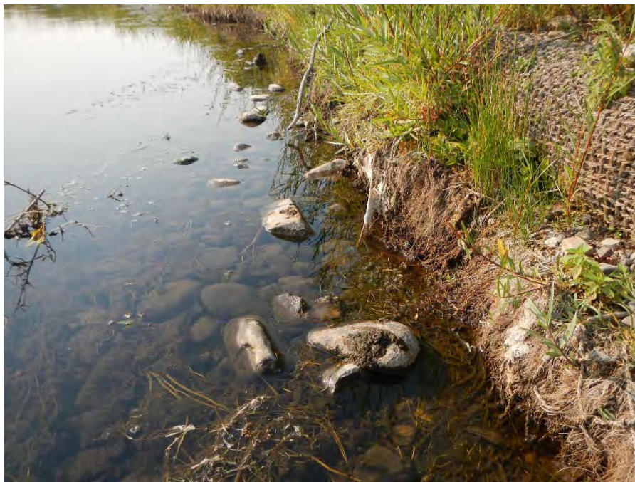
Photo 14. Example of continued fabric decay coupled with vegetative expansion.
