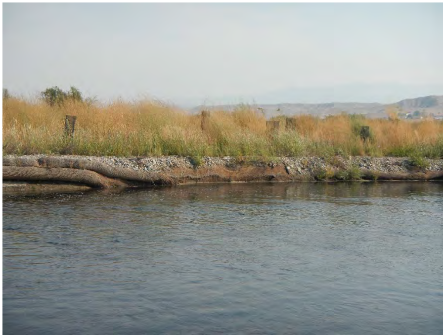
Photo 15. Bank LB-46E identified for continued monitoring.
