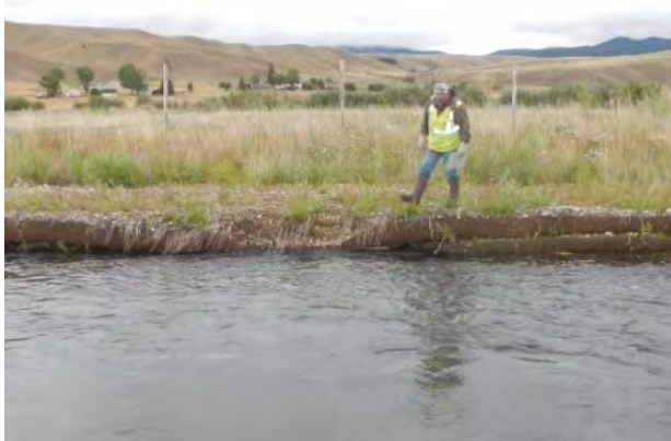
Figure 16. Streambank RB-N-5 with fabric degradation and toe material loss.
