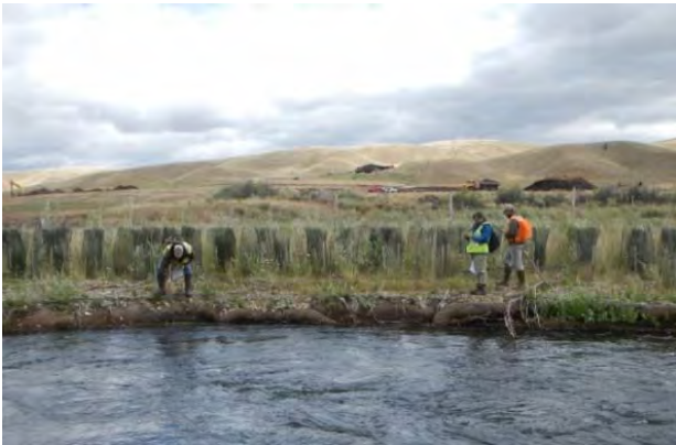
Figure 19. Streambank RB-N-47 DVSL showing fabric degradation and loss of coir logs.
