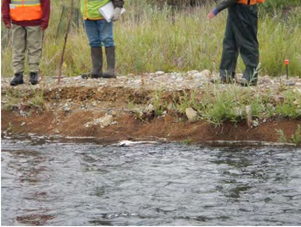
Figure 18. Streambank RB-N-14 DVSL showing loss of coir logs and bank erosion.
