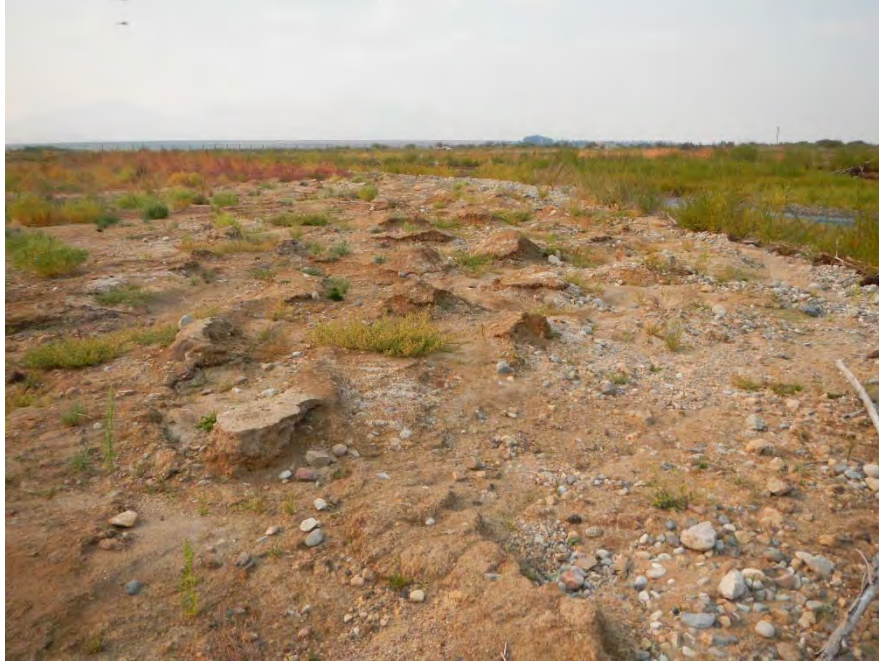
Photo 17. View downstream of floodplain erosion, 85+00L.
