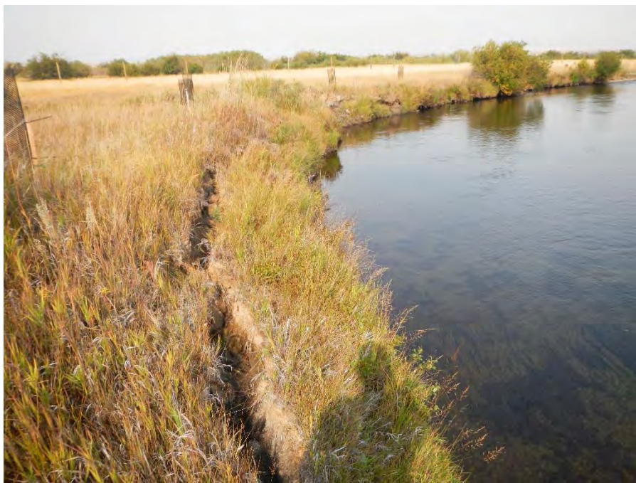
Photo 16. Actively eroding No Treatment bank (LB-40).
