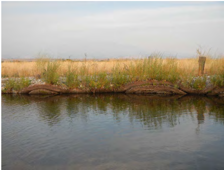
Photo 13. Bank RB-14 identified for continued monitoring.
